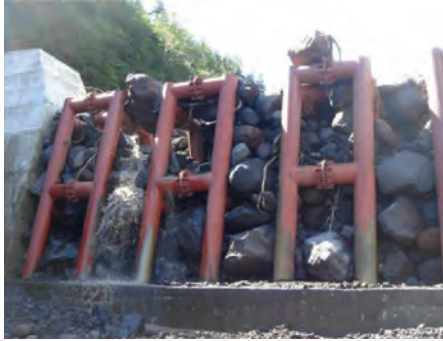
Condition of capturing of debris flow
