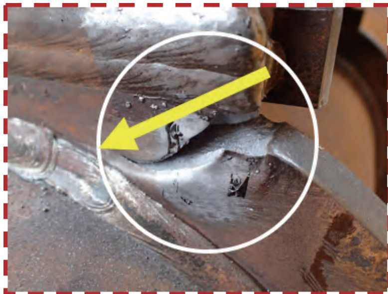
Fig. 7 Fracture of Diaphragm
