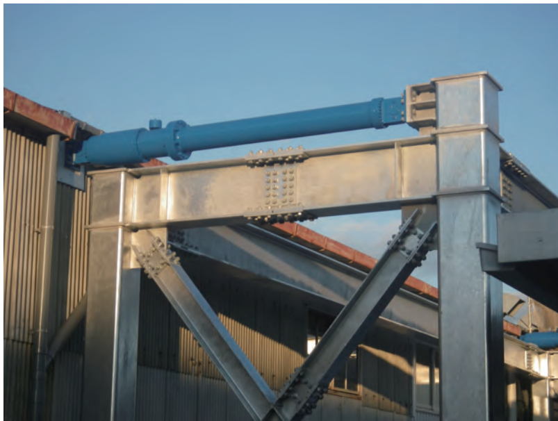
Photo 1 Response-control buttress framing employing viscosity damper
