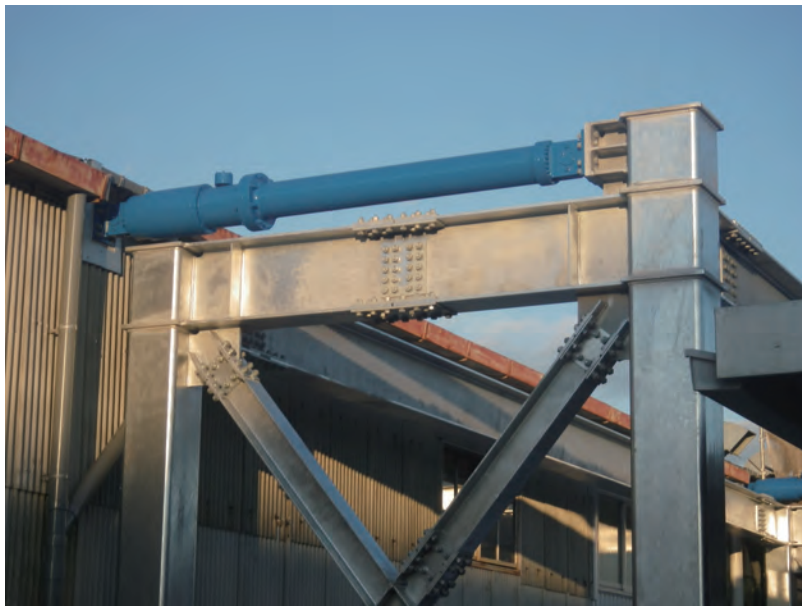
Photo 1 Response-control buttress framing employing viscosity damper
