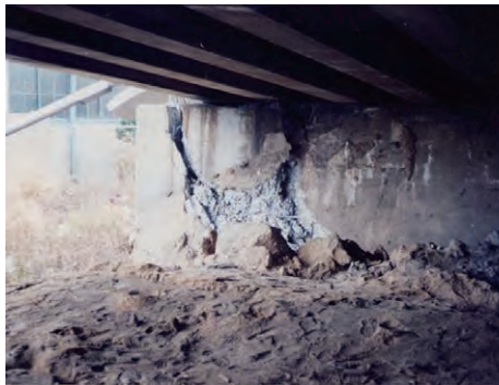
Photo 1 Damage to bridge abutment located in the ground where liquefaction occurred 2)
