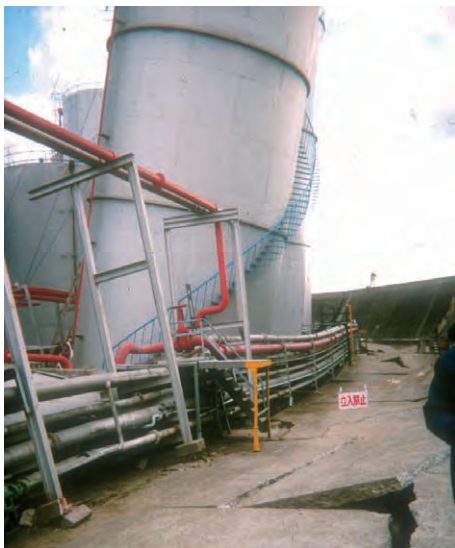
Photo 3 Settlement and inclination of oil product tank by soil liquefaction (1995 Kobe earthquake)
