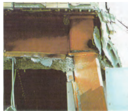
Fracture of column-beam connection
