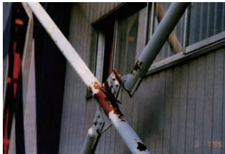
Fracture of brace joint
