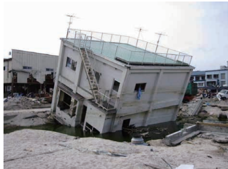
Photo 4 Building that inclined due to scouring
