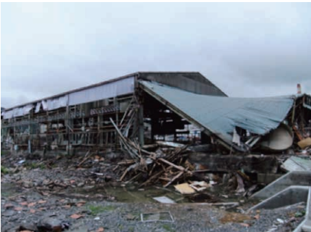
Photo 2 Steel-structure building with which drifts (ship) collided
