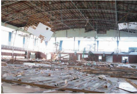
Ceiling members fell due to earthquakes.
