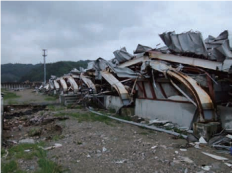
Photo 1 Steel-structure building destroyed by tsunamis
