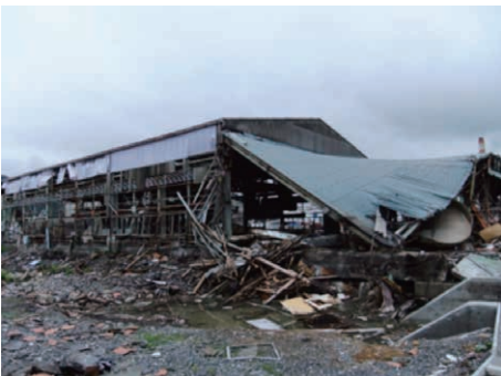
Photo 2 Steel-structure building with which drifts (ship) collided
