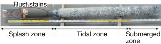
Fig. 5 Appearance of Polyurethane Coating after Rust Removal (23-year Exposure)
