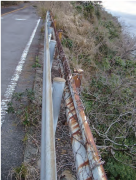
Photo 3 Crush barriers on a disused road as a case of hibernating stock
