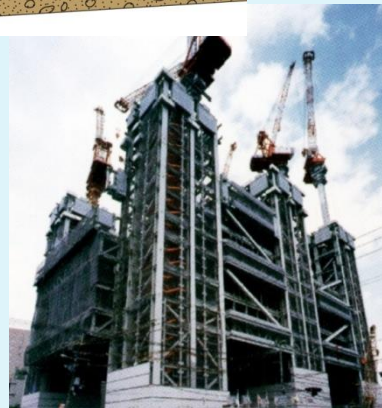
Damping structure by buckling-restraint brace
