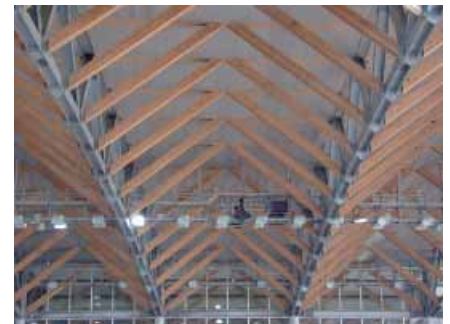
Hybrid truss composed of steel frames and beam and diagonal members made of laminated Kochi Cedar
