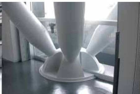
Cast steel member adopted for the space column base
