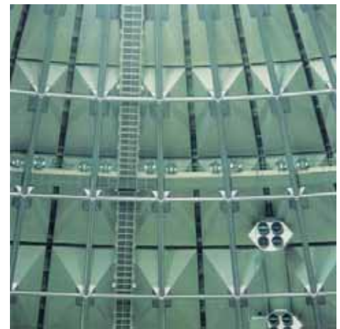
Photo 2 Expanded inside view (the cross-shaped sections are composed of steel castings)
