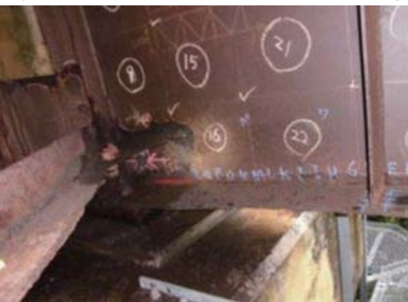
Fig. 4 Three-dimensional Corrosion Map
