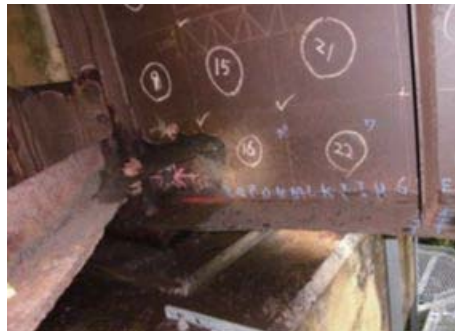
Fig. 4 Three-dimensional Corrosion Map
