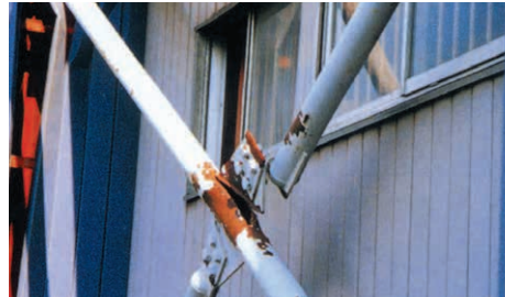
Fracture of brace connection
